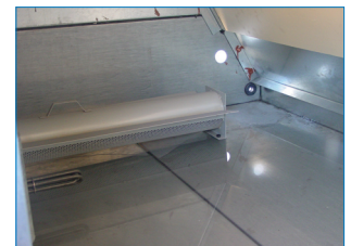
Separate internal cold water basin
