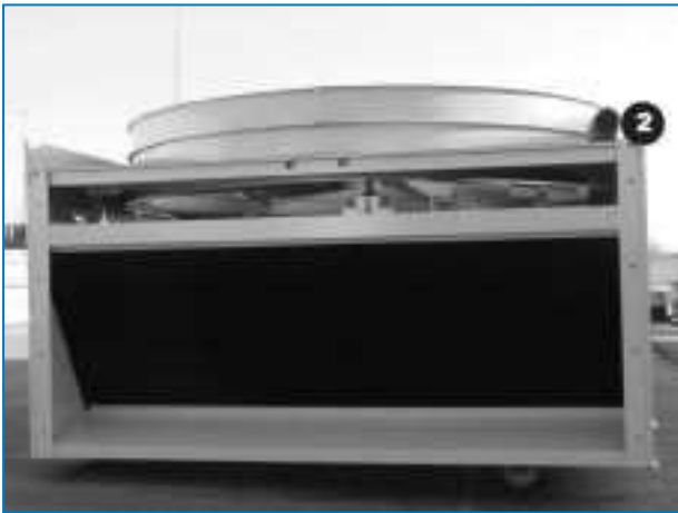
Pump piping connection on plenum section outside
